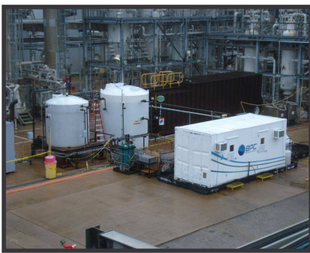
Figure 1: BPC-ACT™ pilot system for treating bilge water
