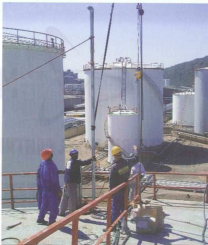
Conversion of accumulated wastewater storage tank to bioreactor
